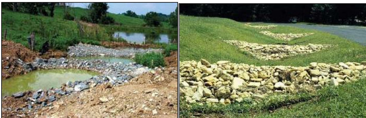
Image 9.1 and 9.2 Example of Silt Traps and Swale with Check Dams to control sediment
