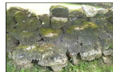
Stone wall on the south eastern side of the turlough. Cinclidotus fontinaloides moss and calcareous deposits indicate that this wall is inundated during the winter months
